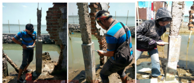
Figure 10. Rebound Hammer Test that was conducted on the retrofitted columns at 12, 13, and 14 months.
