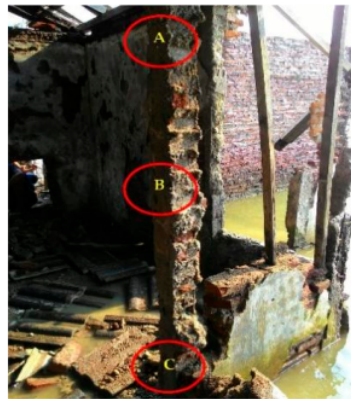
Figure 12. The Rebound Hammer Test was conducted on the points marked by red circles.
