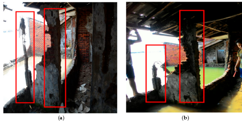
Figure 6. The broken columns which were retrofitted by applying bio-polymer modified concrete, (a) Situation at the time the left column still existed, and (b) Situation in the next few months after the left column had almost collapsed.
