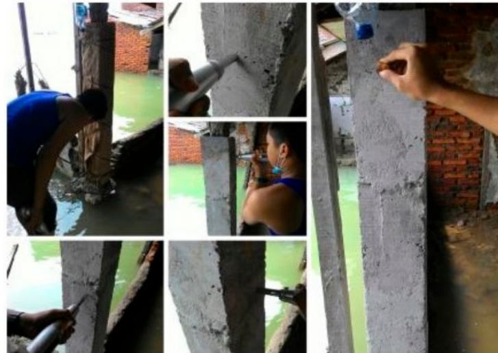
Figure 9. Rebound Hammer Test that was conducted on the retrofitted columns at 7, 14, and 28 days.
