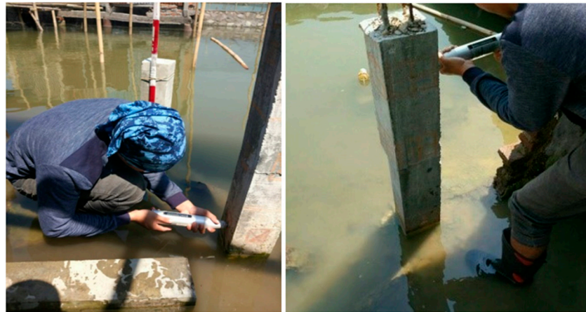
Figure 11. Rebound Hammer Test that was conducted on the control column at 14 months.
