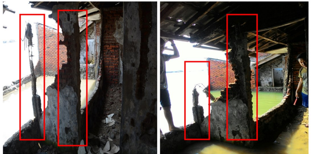
Figure 6. The broken columns at situation of (a) The initial work when the two broken columns still existed, and (b) The next few months after initial work when the half part of left column had been collapsed.
