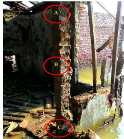
Figure 12. The Rebound Hammer Test was conducted on the points marked by red circles.
