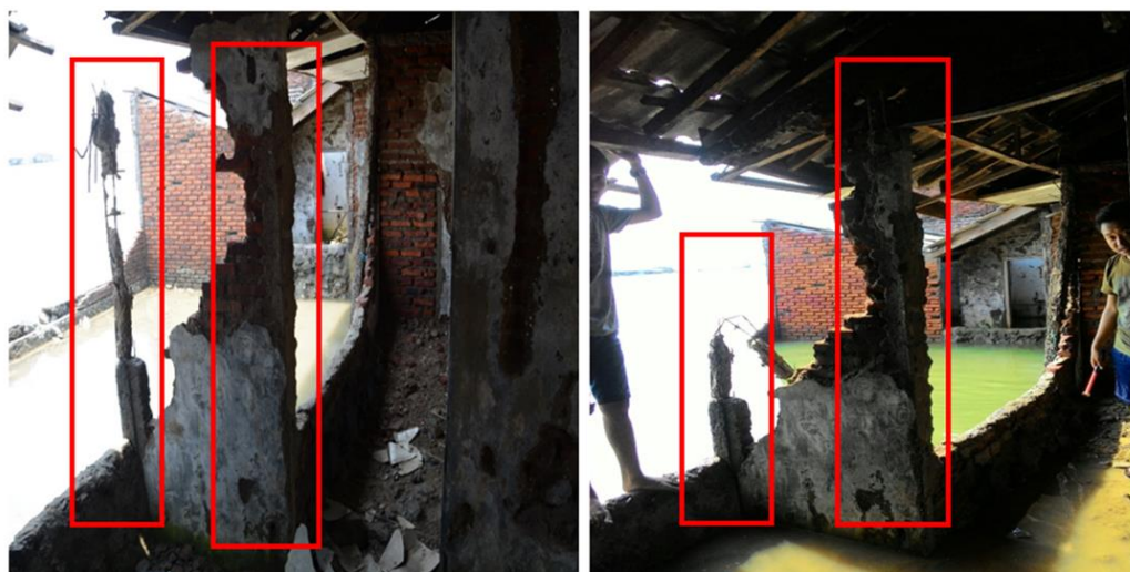
Figure 7. The broken columns which were determined to be retrofitted by applying bio-polymer modified concrete; (a) Situation at the time the left column still existed; and (b) Situation in the next few months that the left column had been almost collapsed.
