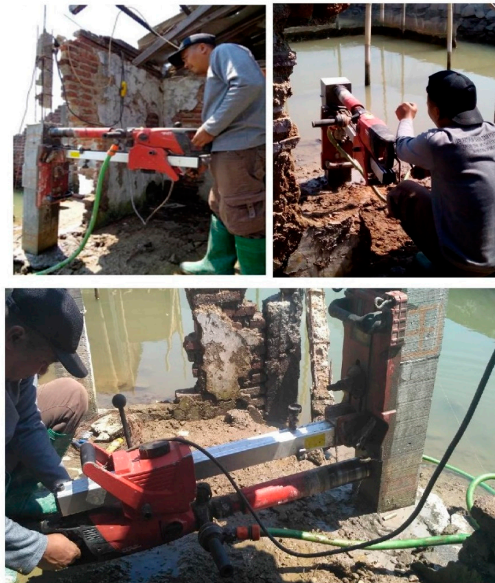
Figure 18. Core Drill method of retrofitted and control columns conducted to obtain samples used for the compressive strength test.
