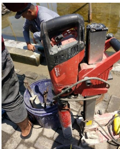
Figure 4. The Core Drill method was using HILTI DD 150-U machine with versatile diamond drilling
