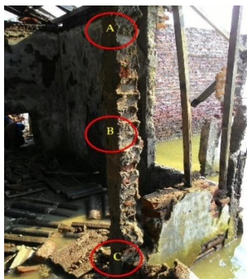
Figure 12. The Rebound Hammer Test was column at conducted at the points that marked by red circles
