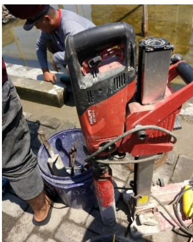
137 138 139 140 Figure 4: The Core Drill method using HILTI DD 150-U machine with versatile diamond drilling
